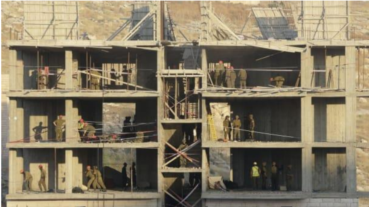
Israeli forces demolish a building at Sur Baher near the separation barrier, July 2019. Credit: Mahmoud Illean / AP
